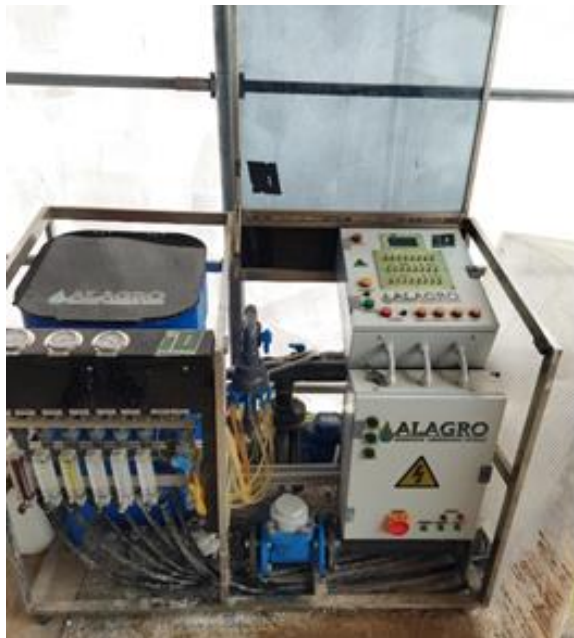
Figure 7: Monitoring and control unit.
